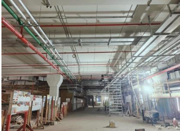
Fire Pipe & Water Supply Pipes Installed
