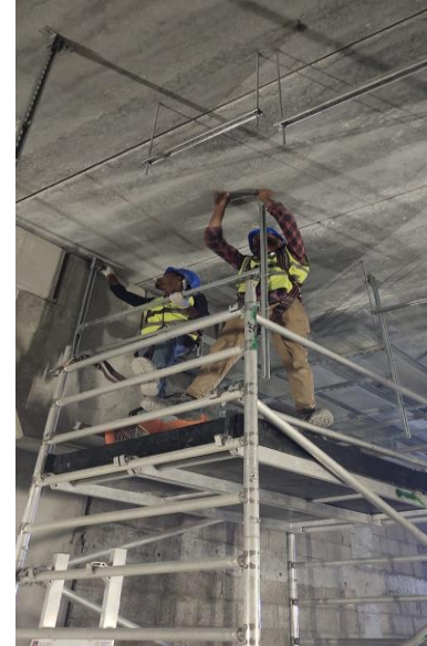
Installation Support for Cable Tray
